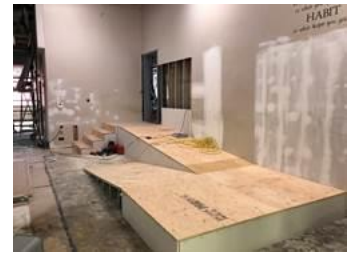
On the north end of the gym, this is the access to the displaced offices from the expanded spin room.
