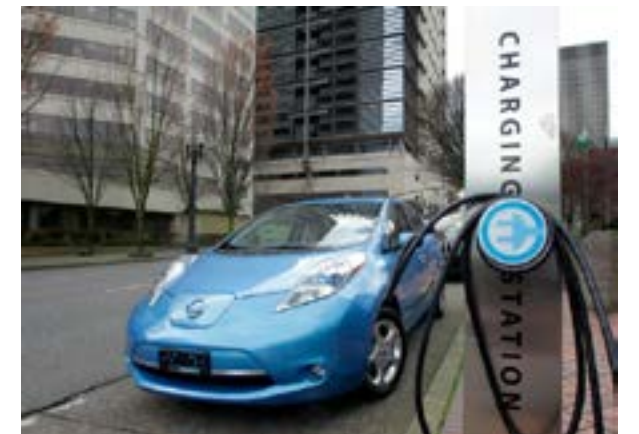
Example of an electric vehicle charging station
